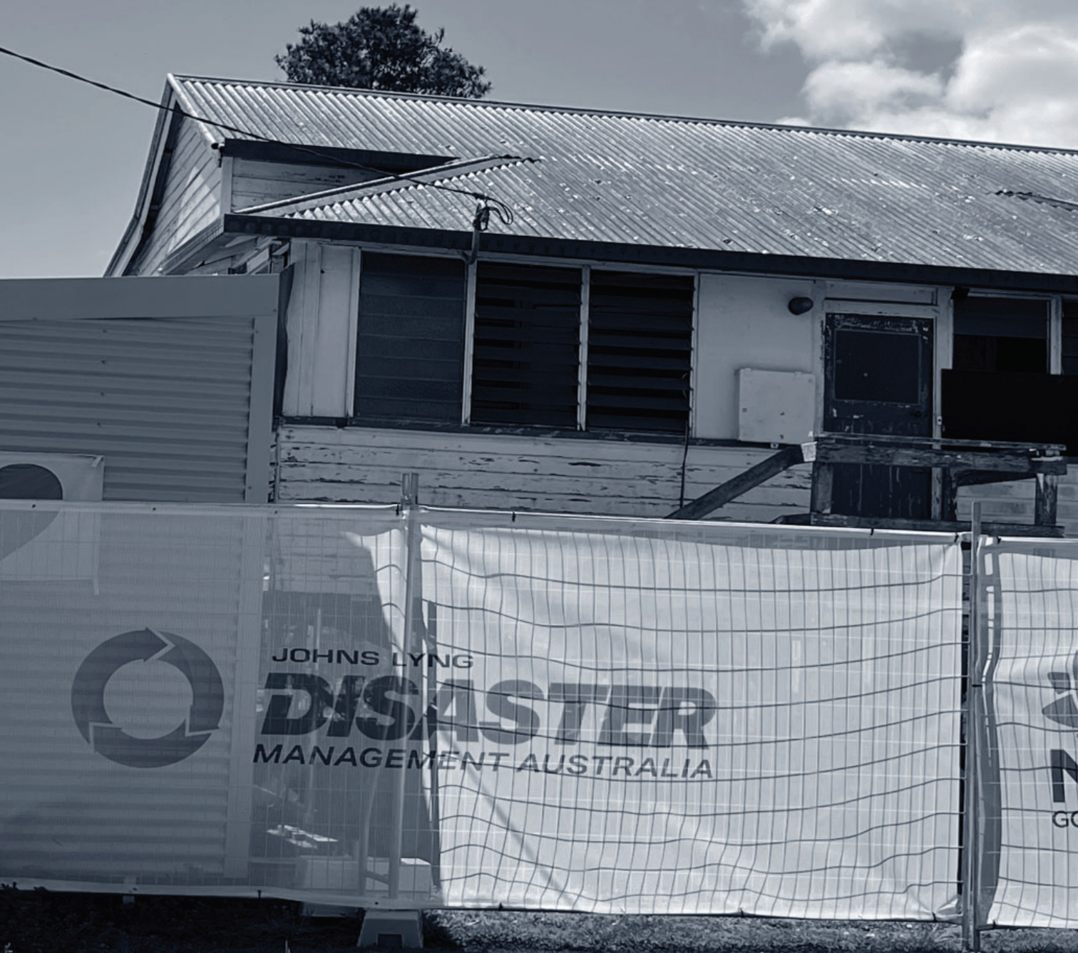
Fig. 12. One of Many Damaged and Unliveable Houses six Months After the 2022 Lismore Floods
